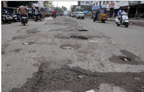
Fig 3.1 Damaged road with pits and holes
